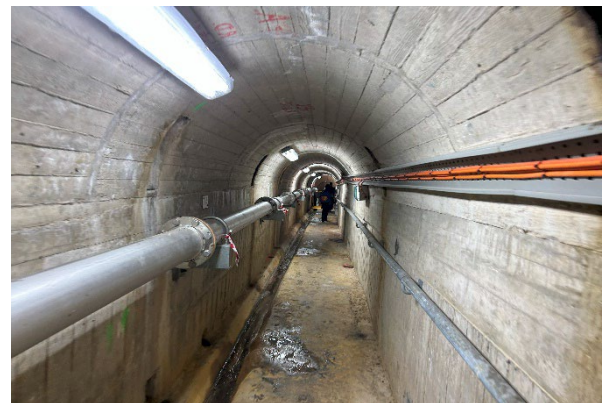
Figure 8: The inside of the Glenmaggie Weir where staff monitor and operate the floodgates.
